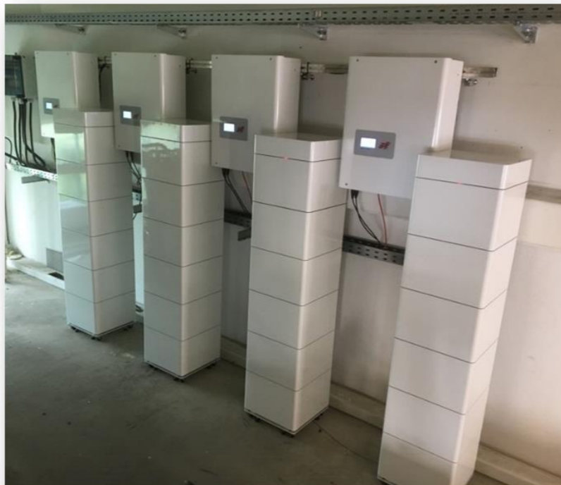
Power Storage AC 6.0 41,6 kWh 100 kWp
