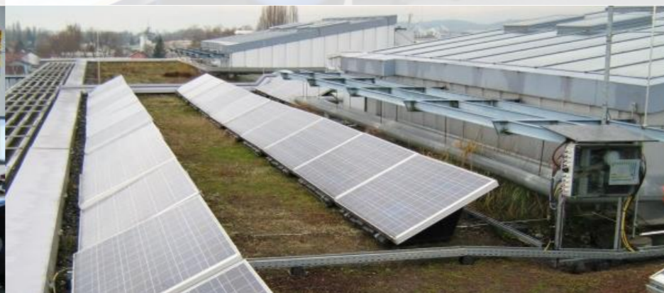
PV Installation - 9 kWp
