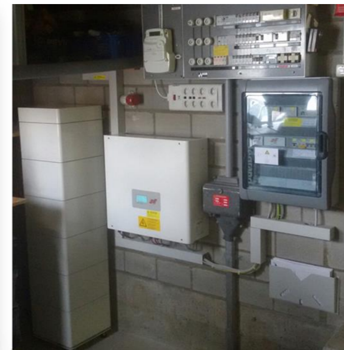
9 kWp – 11.5 kWh Storage DC 6.0 and Power Switch
