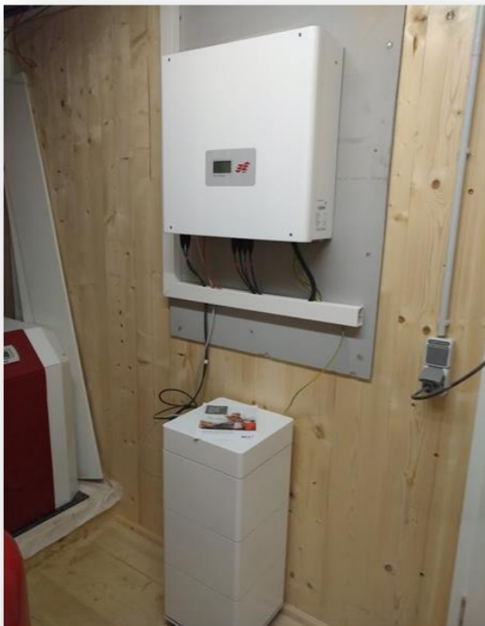
6.4 kWp – 5.7 kWh Power Storage DC 6.0
