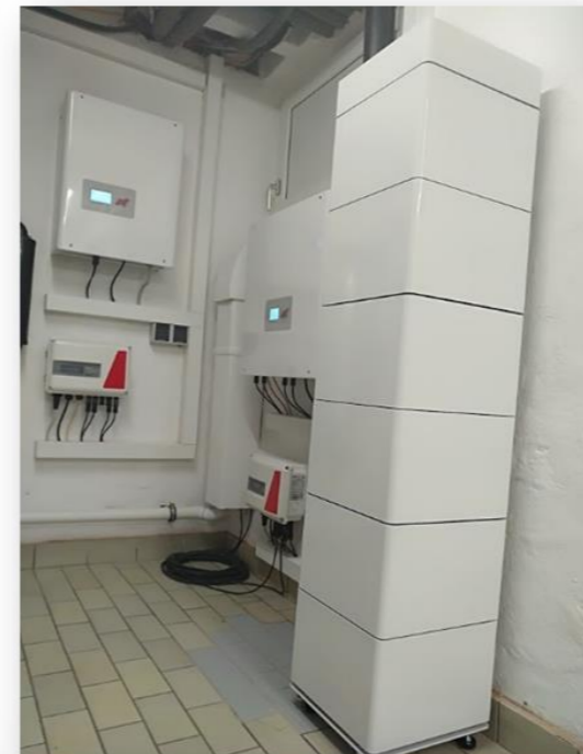
Power Storage DC 6.0 and Inverter 4.0 12 kWp – 11.4 kWh EV charger for BMW i3
